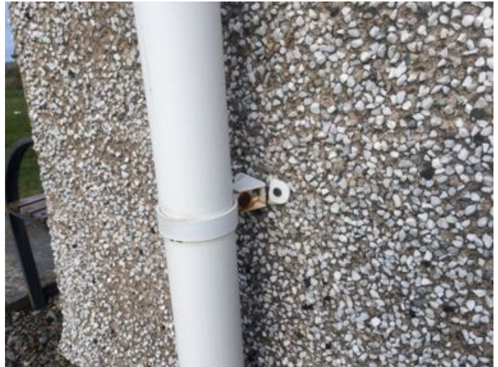
Broken gutter bracket West elevation
