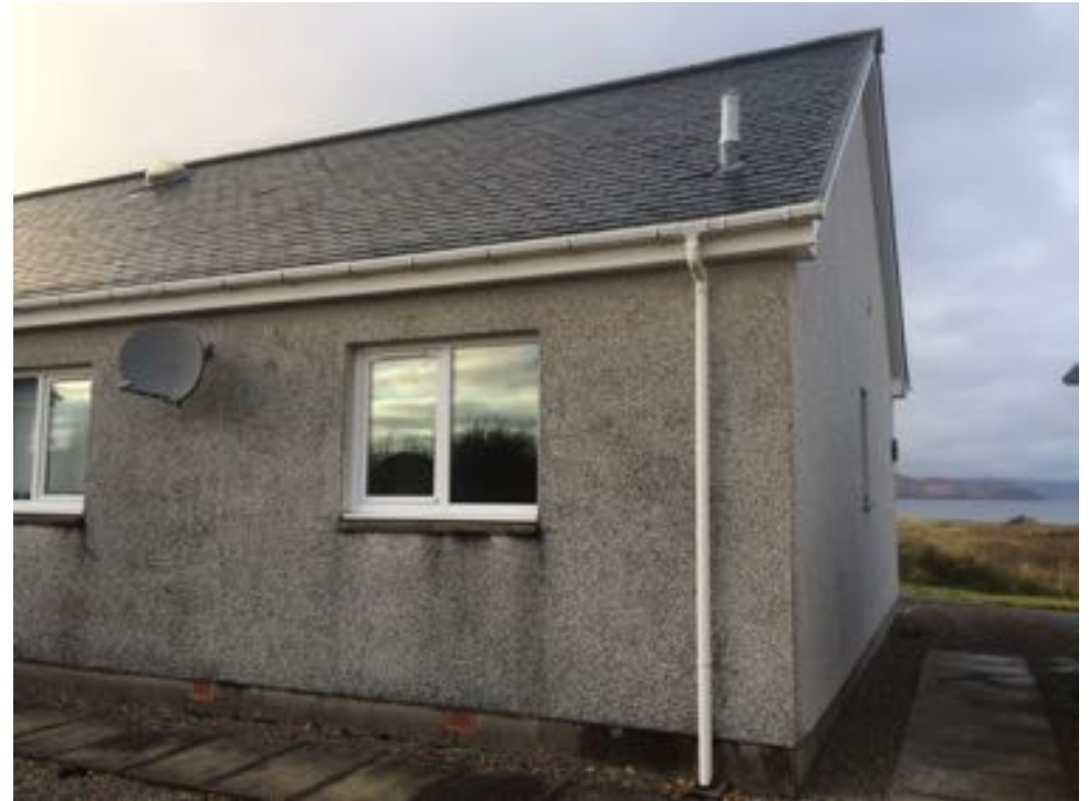
External damp stain at rear window
