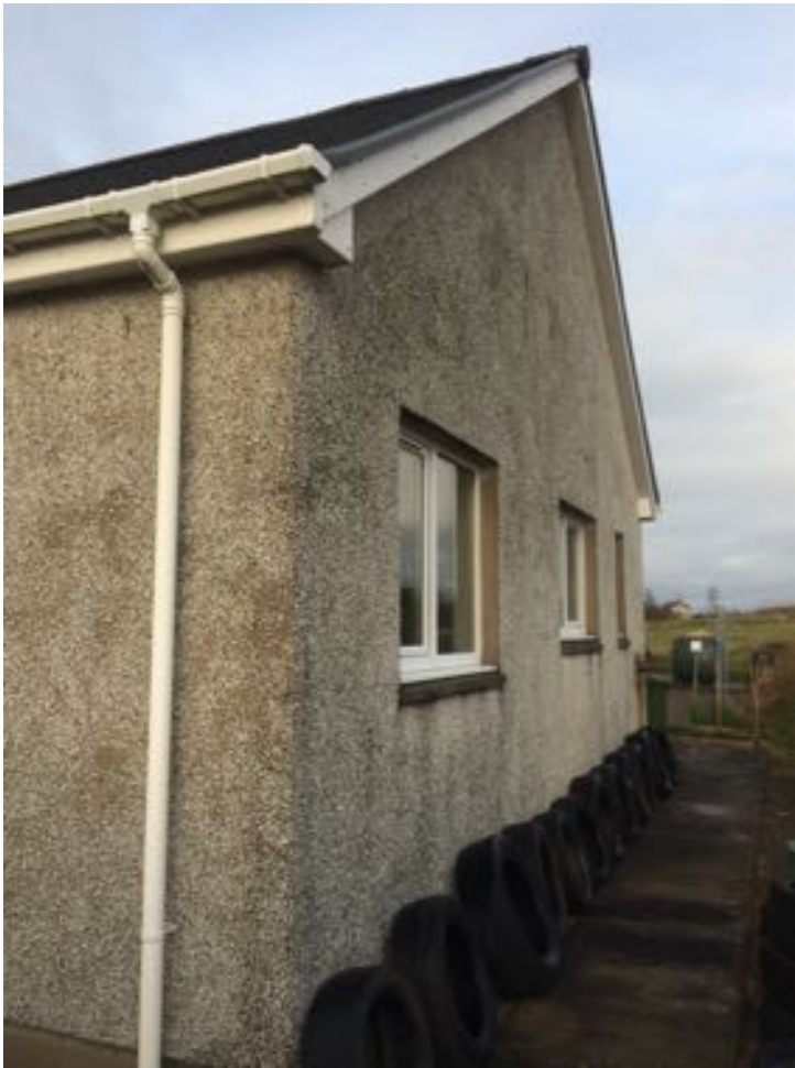
Rear elevation South East gable showing worn dry dash render
