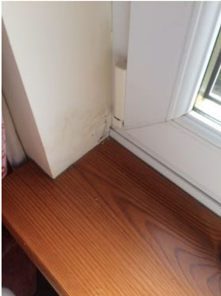
Damp ingress at corner of window in bedroom 3
