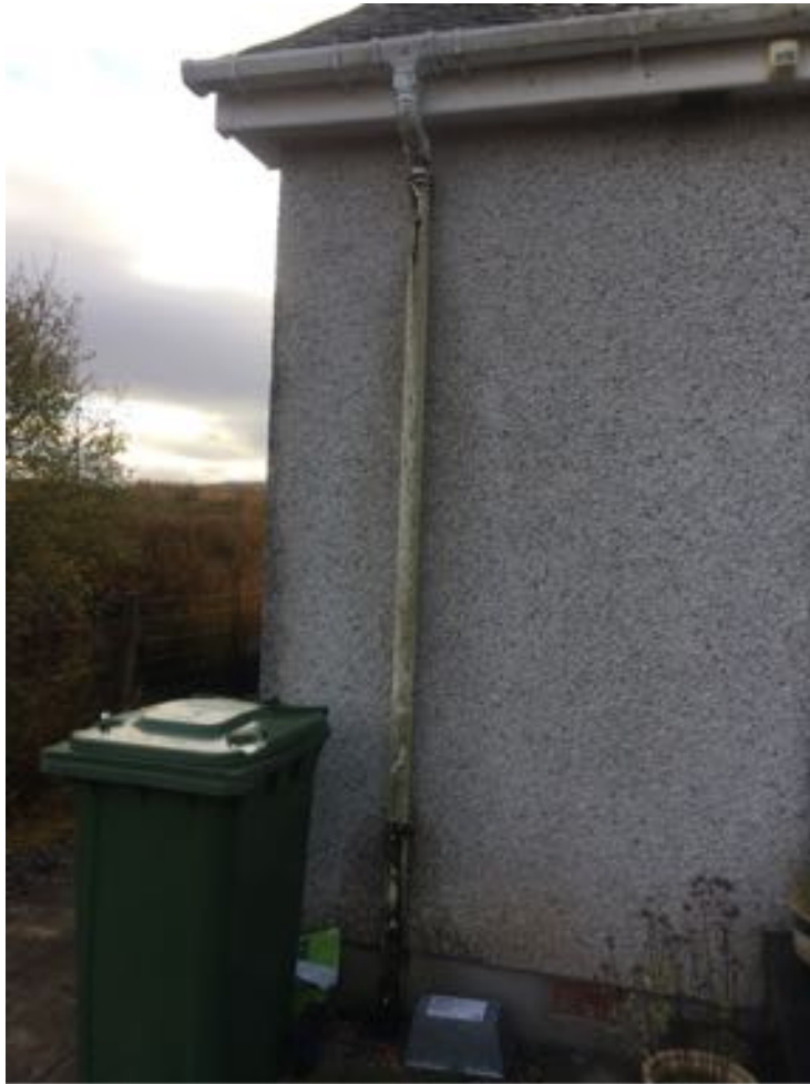
Downpipe at South East corner showing algal growth
