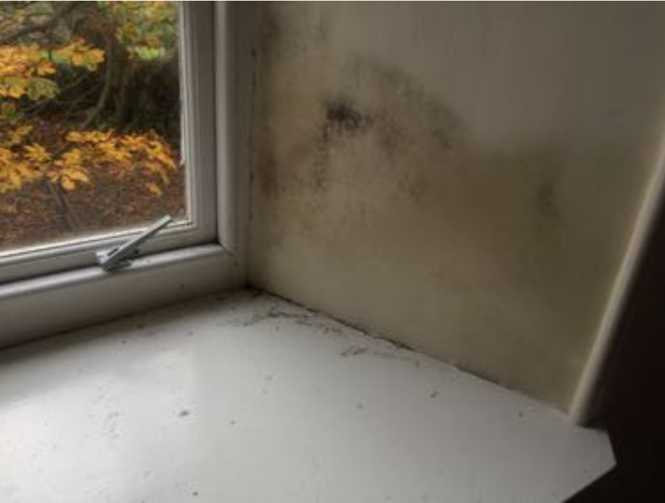
Dampness at South facing window in vestry
