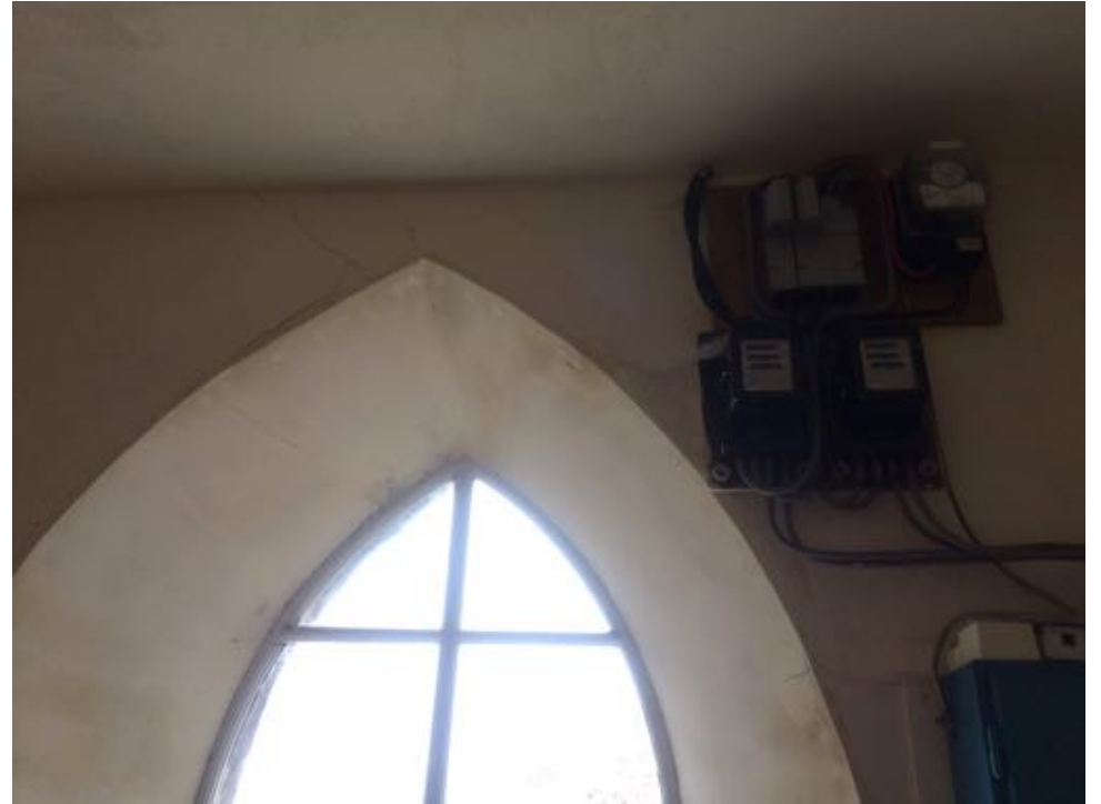
Dampness and cracking adjacent to window in vestry
