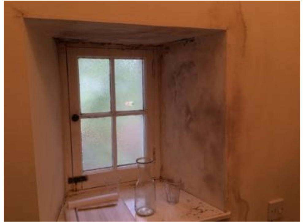
Dampness in external wall of rear w.c.
