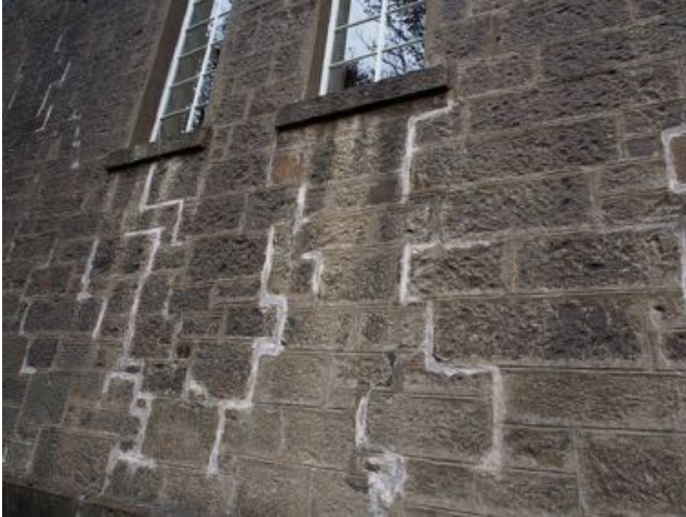
Cracks in South gable pointed up
