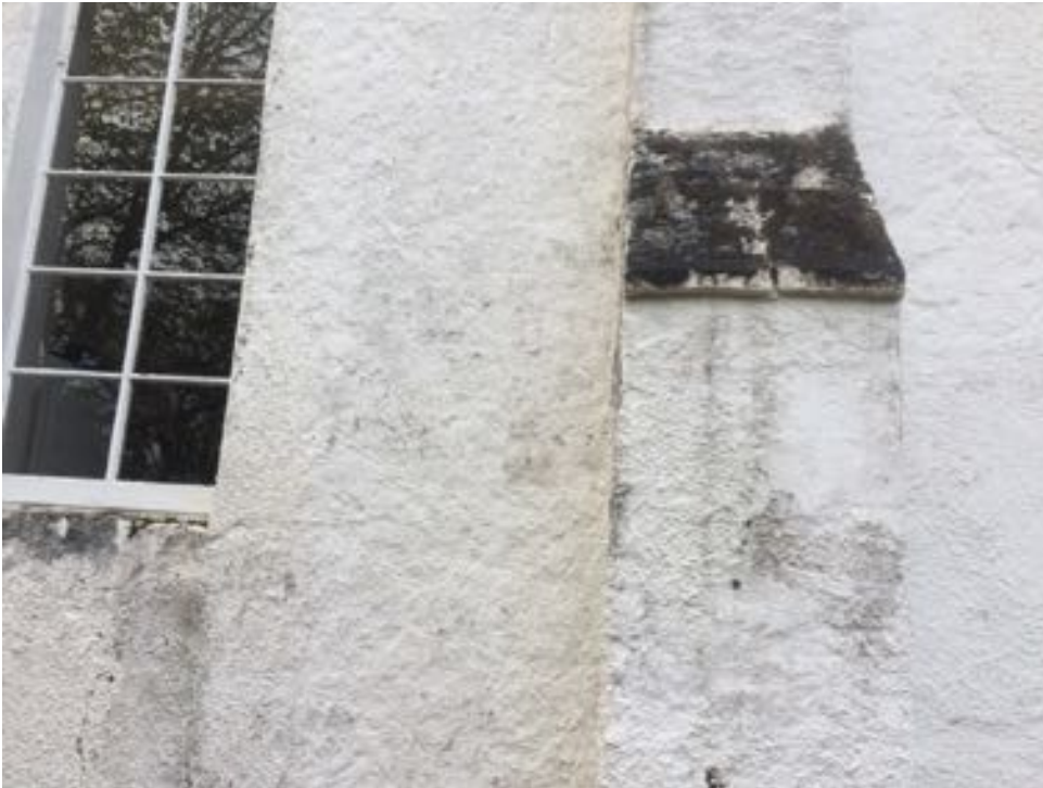
Buttress on East elevation, note note damp on sloped surface and crack under window
