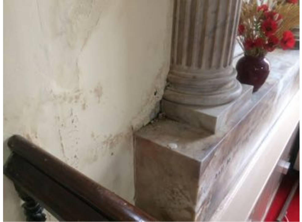
Dampness in wall adjacent to monument on right hand side of pulpit
