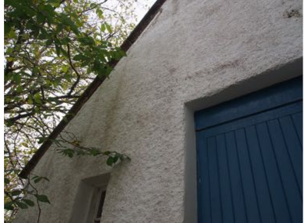
North side of lean-to showing gaps in skew and defective render
