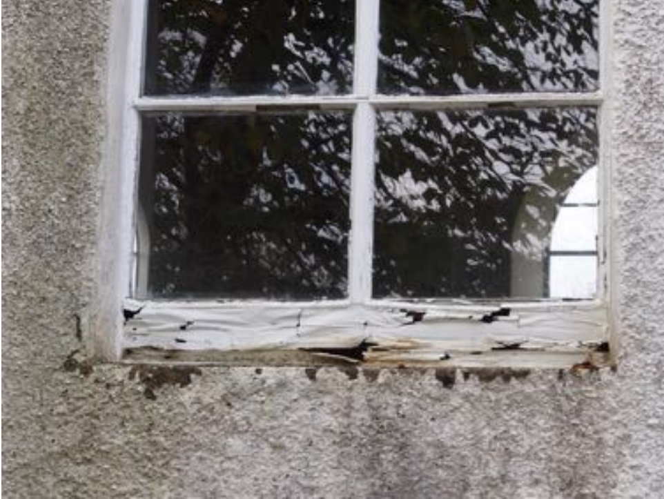
Rotten bottom rail to window on East elevation, note flat window ledge without cill to shed water
