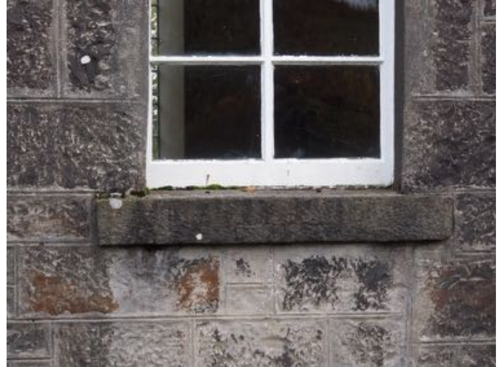
Window cill on West elevation is very flat and has some moss growth
