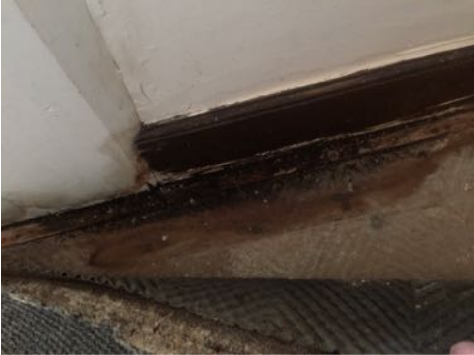
Dampness affecting floor and wall below window in vestry
