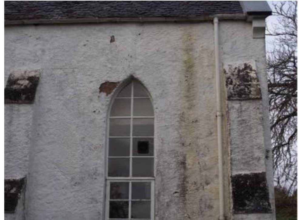
Defective render and crack above window, damp staining from defective gutter on East elevation
