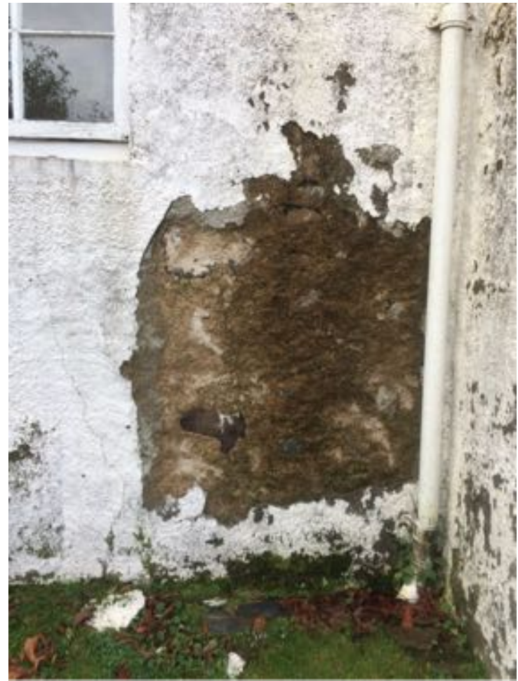
Defective render on East elevation
