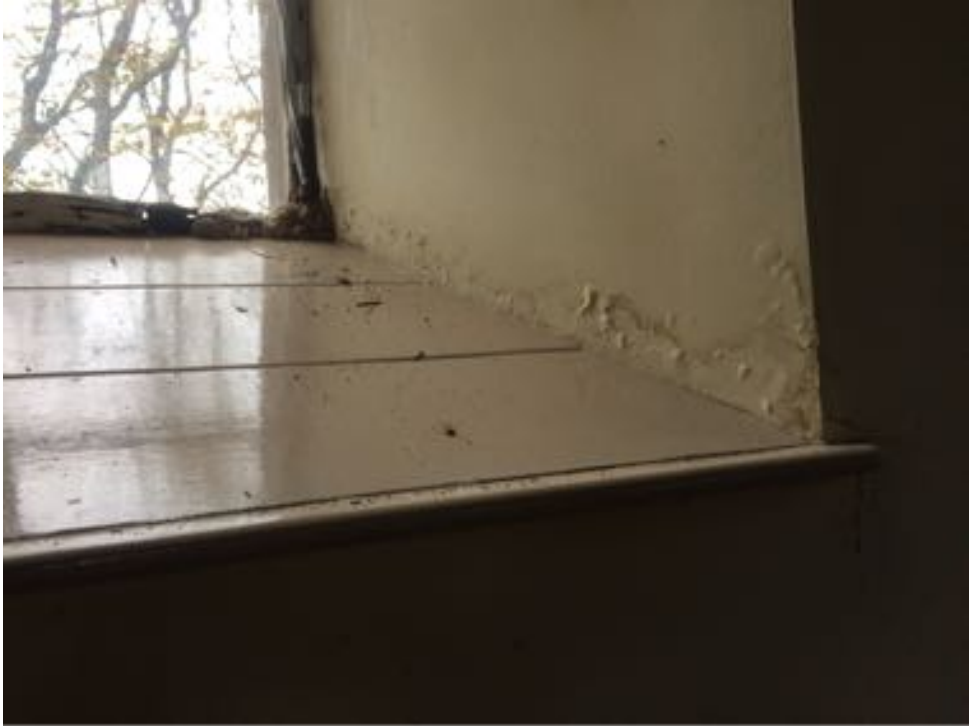
Defective window frame and water ingress at base of window on South gable
