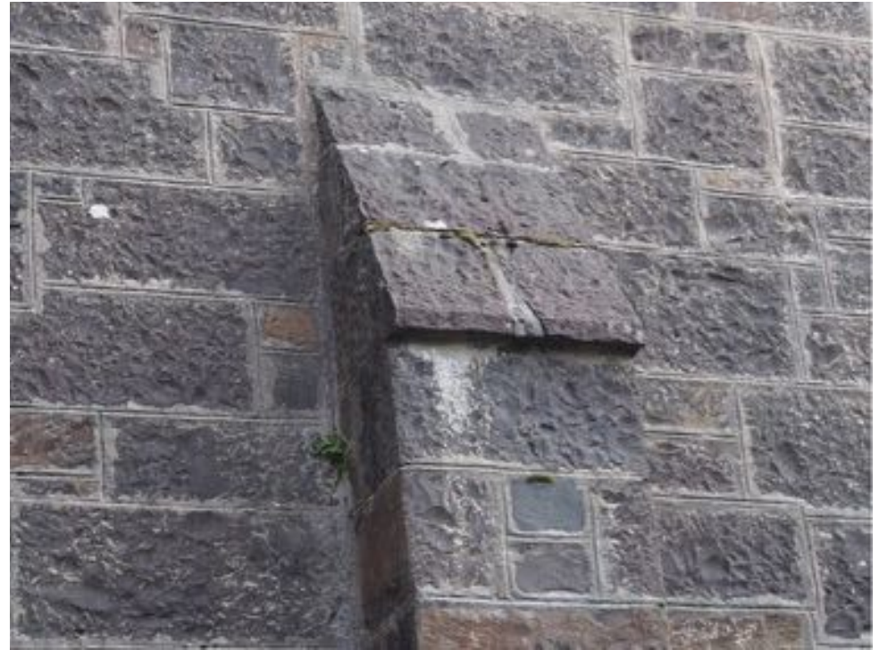
Top of buttress showing slight defects to pointing and moss / vegetation growth
