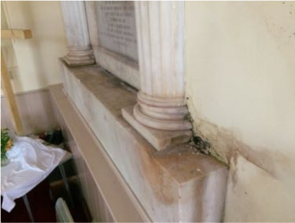
Dampness in wall adjacent to monument on left hand side of pulpit
