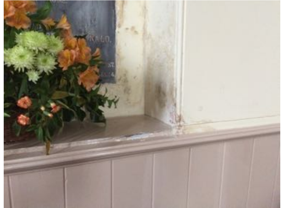
Dampness in wall at niche on west elevation. Note buttness is immediately behind the alcove
