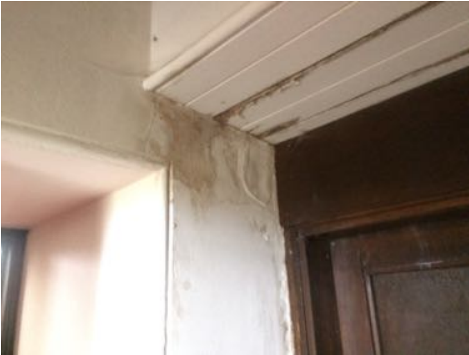
Dampness over external door and w.c. door in lean-to, associated with pointing to skew and render on external wall above
